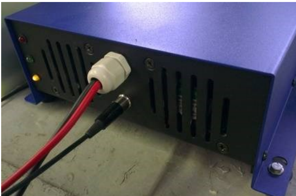
BMS-Charger signal cable plugged into the Charger; yellow LED light is ON-Charger is working
